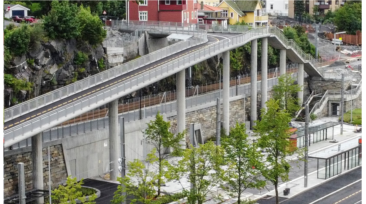
Substation placed neatly as part of a concrete and dry wall construction at Fløen, line 2
