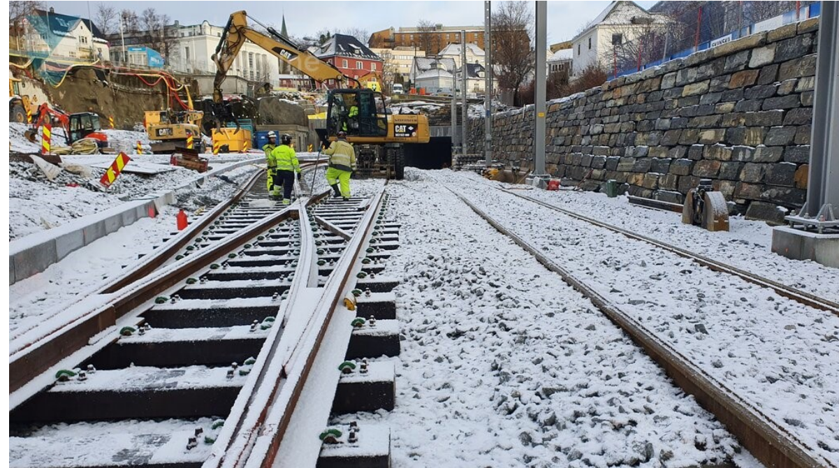
Track switch at Kronstad line 2
